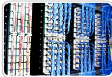
UTP patch panels in a rack
